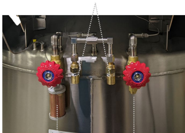
Pressure Relief Valves
