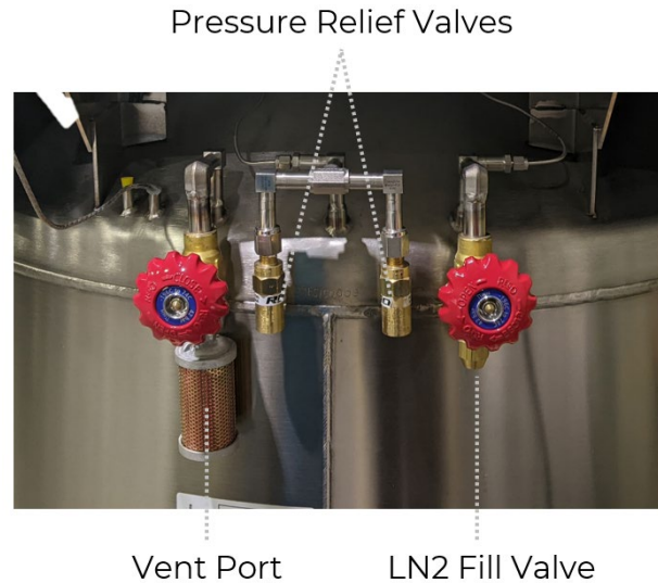
Figure 19: Vent port, dual Pressure relief valves, LN 2 fill valve
